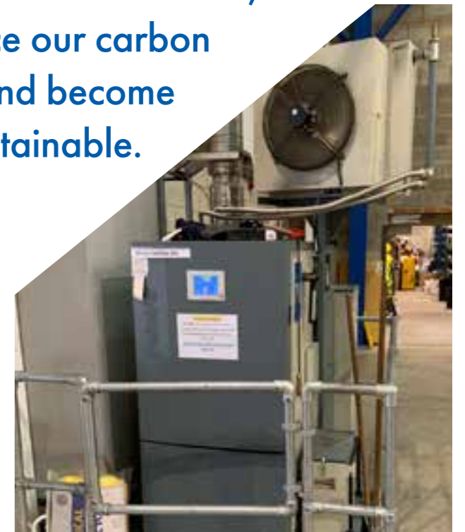
Northampton Biomass Boiler
